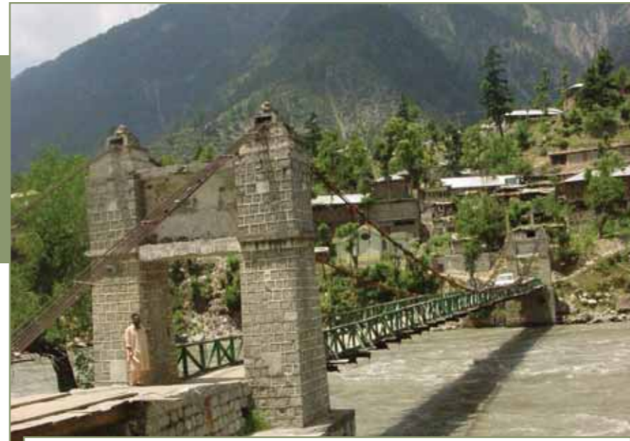
"This rickety bridge with missing planks and snapped support lines bears the scars of cross-border firing. Before the ceasefire, Bun Chhattar would be cut off from the outside world for days on end."
